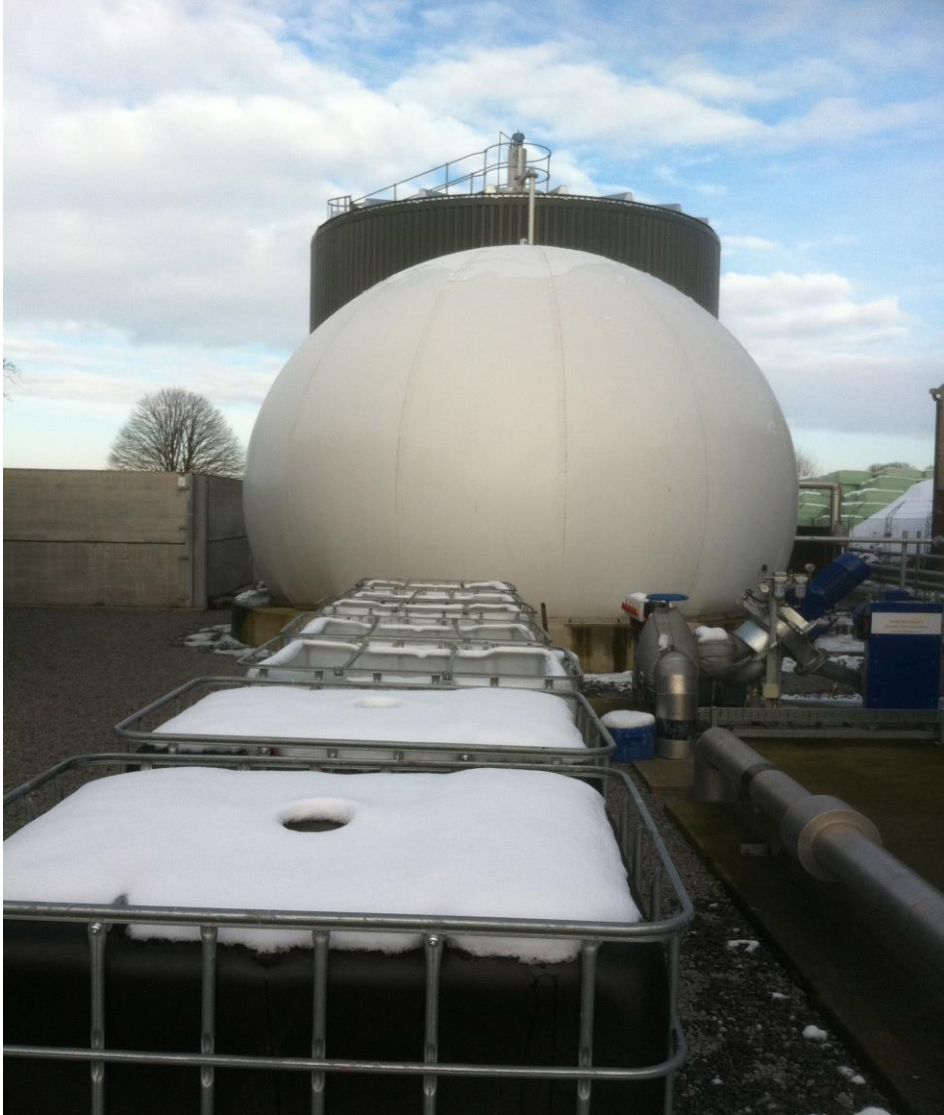
Reaseheath College Anaerobic Digestion Facility
